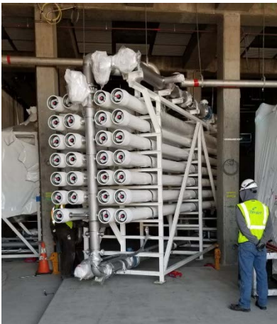
Caption: One of eight skids being set in place at the Westside Recycled Water Treatment Facility, San Francisco in California.
