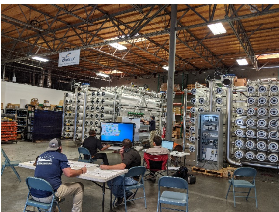
Caption: Factory acceptance testing area at Biwater's facility in California.
