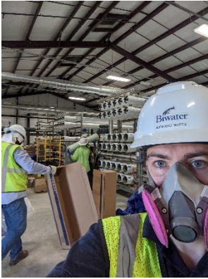
Caption: Membrane loading at the City of Goodyear, Arizona.
